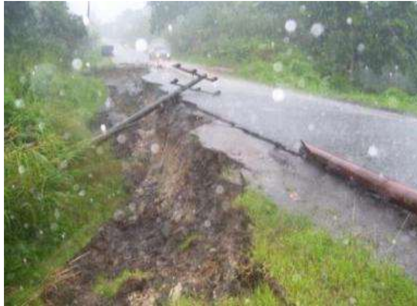
Landslide in Padang, Sumatera Baraf after Earthquake in 2009 Faizal, 2009
