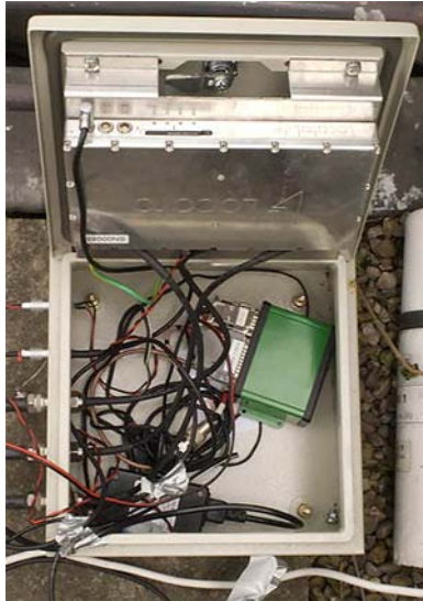
Figure 4 Locatalite with Datalogger attached
