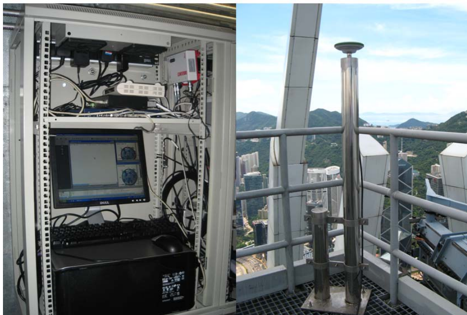
Fig 13: GNSS monitoring in the IFC2 tower in Hong Kong
