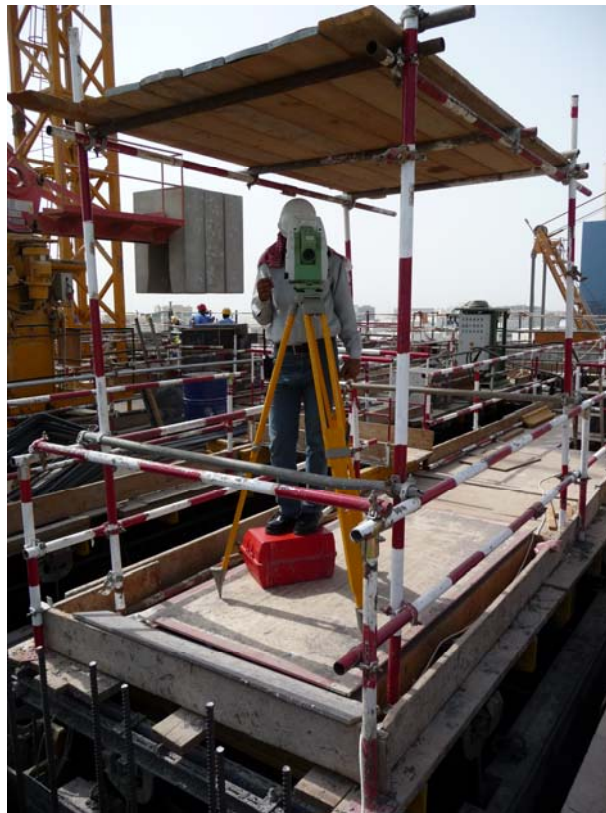
Fig 9: typical setup of a TPS on top of high-rise building in Kuwait
