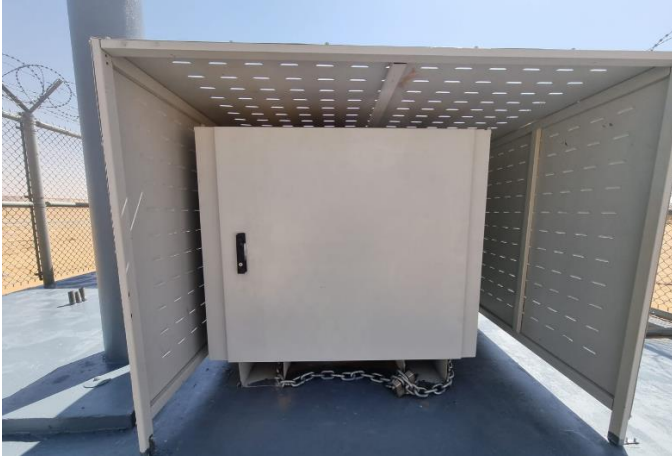
Figure 6: KSA-CORS Cabinet protective layer
