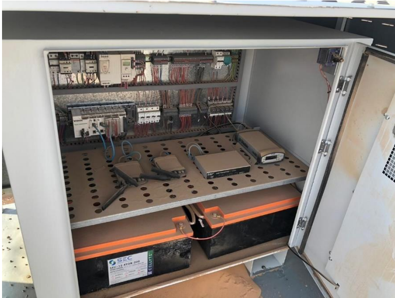
Figure 2: : KSA-CORS IP66 Internal Cabinet filled with Dust
