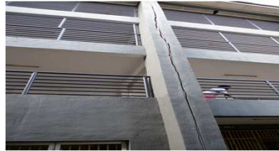
Fig 4: crack along outside Column D4
