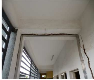
Fig 5: Crack around Beams
