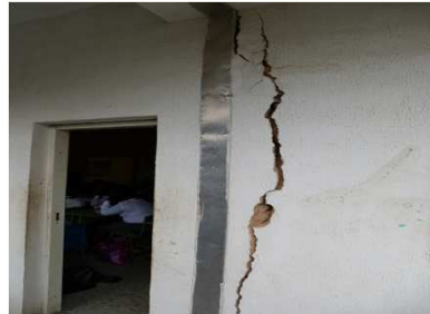
Fig 6: major crack in wall
