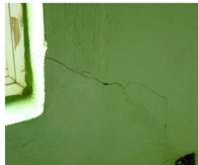
Fig 8: crack in Window
