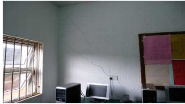
Fig 3: crack in office wall
