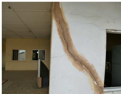
Fig 7: diagonal crack on wall
