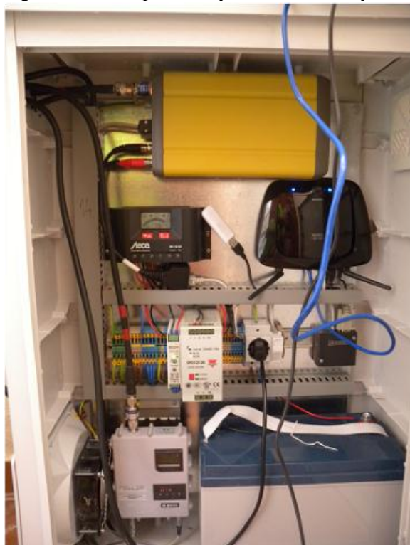
Figure 3 – Example of a system installed by SEGAL (Angola)
