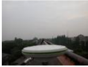
Figure 5. Leice GNSS antenna belongs to ITB CORS which has been installed at the top of Geodetic Department, ITB, Bandung
