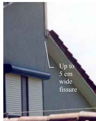
Figure 12: Picture of fissure in a house near to point 204
