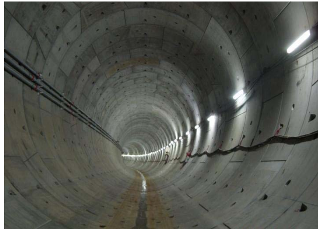
Figure 2 The lining of the tunnel is formed by a continuation built up of the rings
