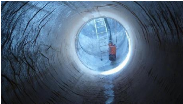
Figure 10: Creasing of liner on clarifier 4
