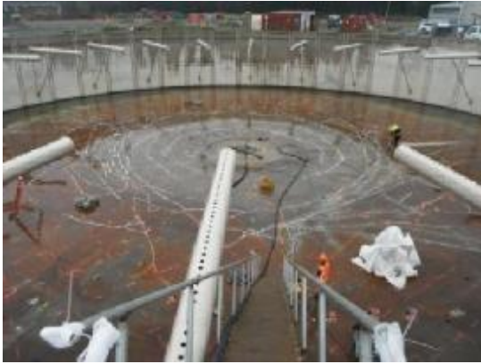
Figure 6: Inverted floor cone on Clarifier 3
