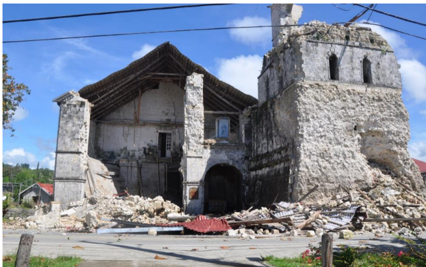
Figure 1: Photograph of damaged Baclayon Church taken during the conduct of GNSS The survey campaign.
